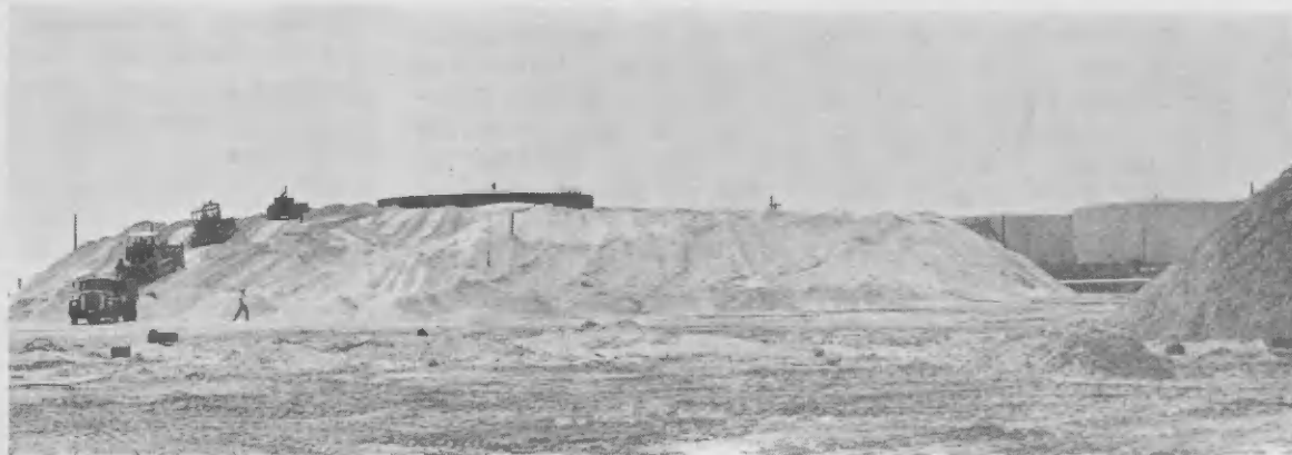
Trucks and tractors resemble crabs on this huge pile of sand, 25 feet high, used to compact the subsoil for tank foundations.
